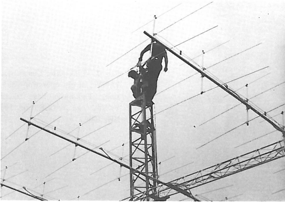
Fig. 10. Only 10 feet to go! The 144 MHz 160-element col-linear array of W4DFK being hoisted into position. W4UPJ and W4UGE are working on the tower.
